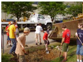
Boy scouts at the Defense Supply Center Richmond construct a rain garden (bio-filtration area) to trap and filter runoff from an adjacent parking lot.
